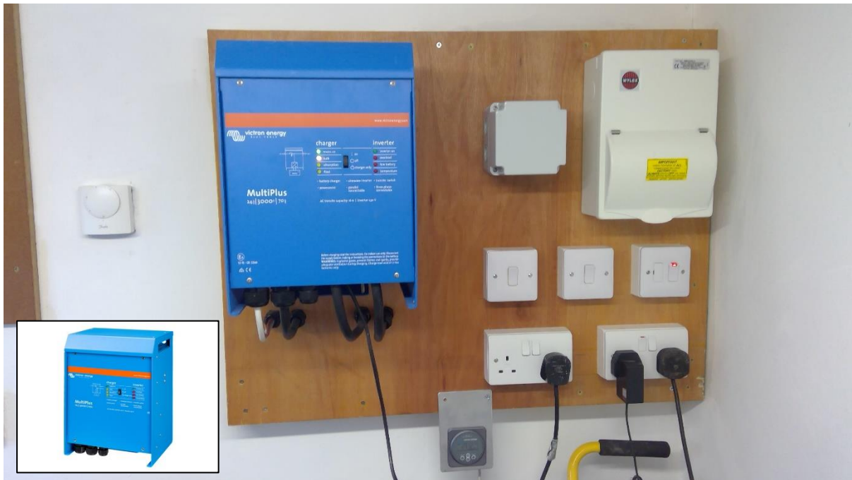
Figure 2 Victron MultiPlus Inverter Charger 12V/3000VA/120A, and installed.
